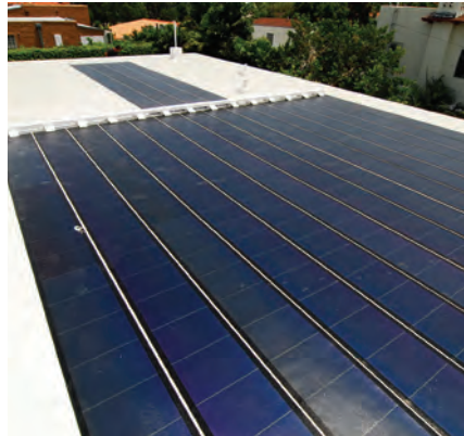
Thin film flexible PV panels on rooftop. Photo Ken Fields, Creative Commons
