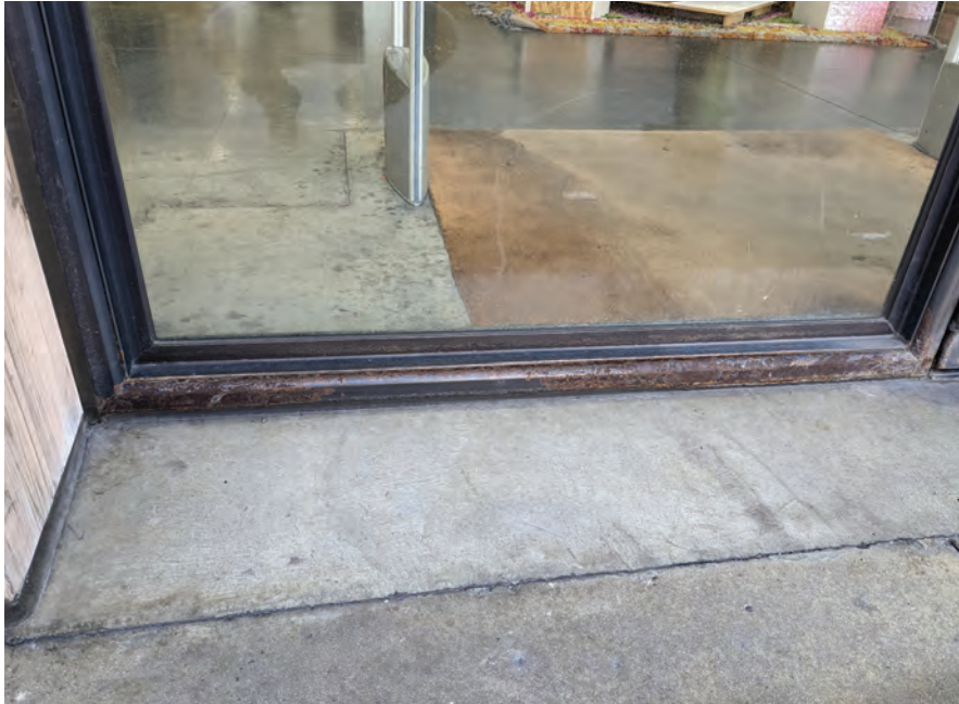
Example of finish damage on a commercial building due to chemical moisture.
