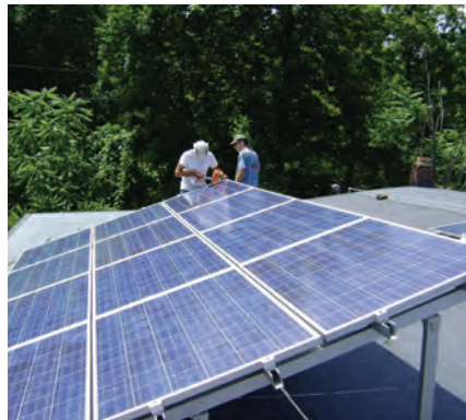
Tilt-up solar PV module array on rooftop. Photo Lucas Braun, Creative Commons
