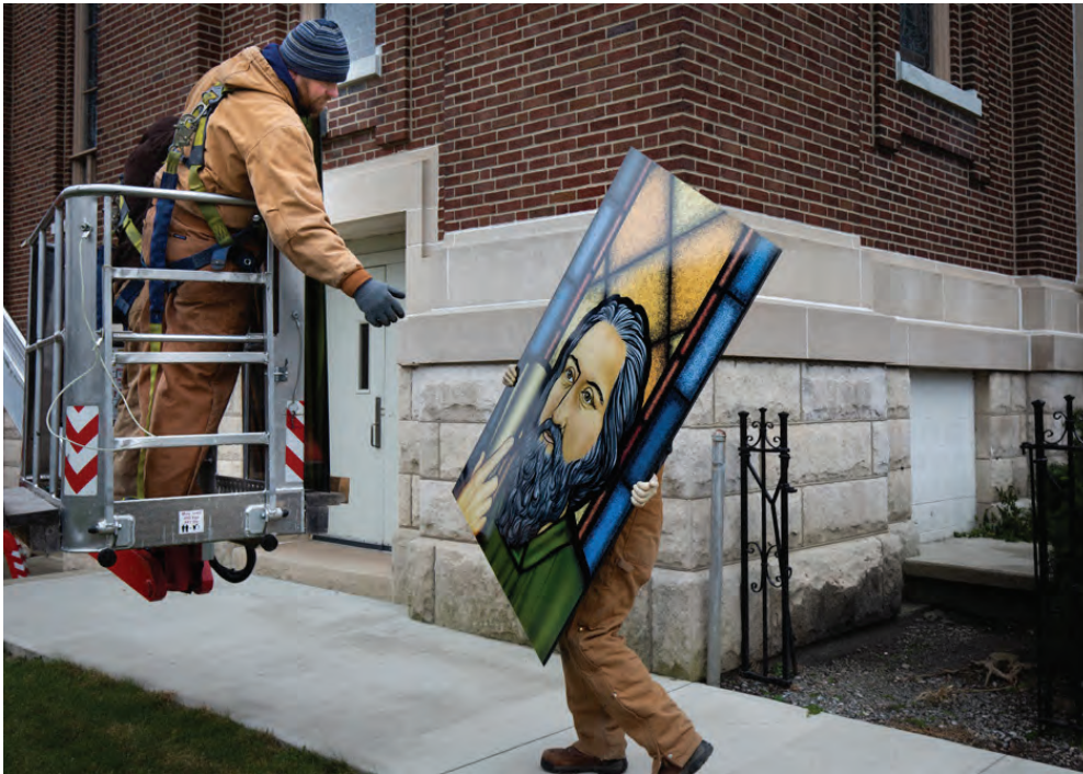
Example of handling a decorative glass lite during installation. Photo courtesy of Window Creations and Vibrantz Technologies.
